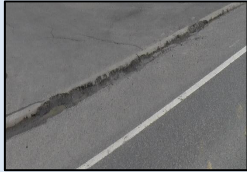
Broken curb at the rear driveway of Dollar General on State Route 31
