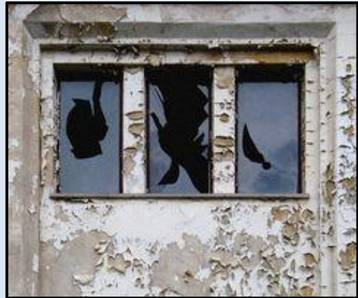
Example of a typical building code violation- building in a state of disrepair/safety hazard
